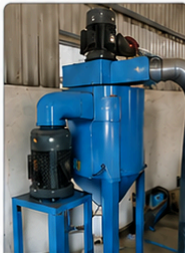
DUST COLLECTION SYSTEM
